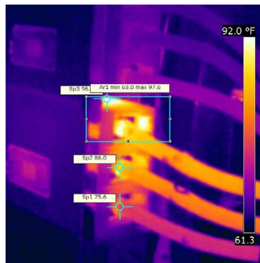
Fig 5 – Temperature Differences between Three Sockets
